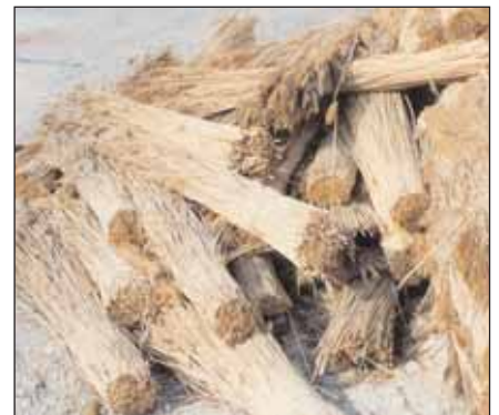
Traditional thatching, photos from top: Reed bundles, building a ridge roll and reed thatching
