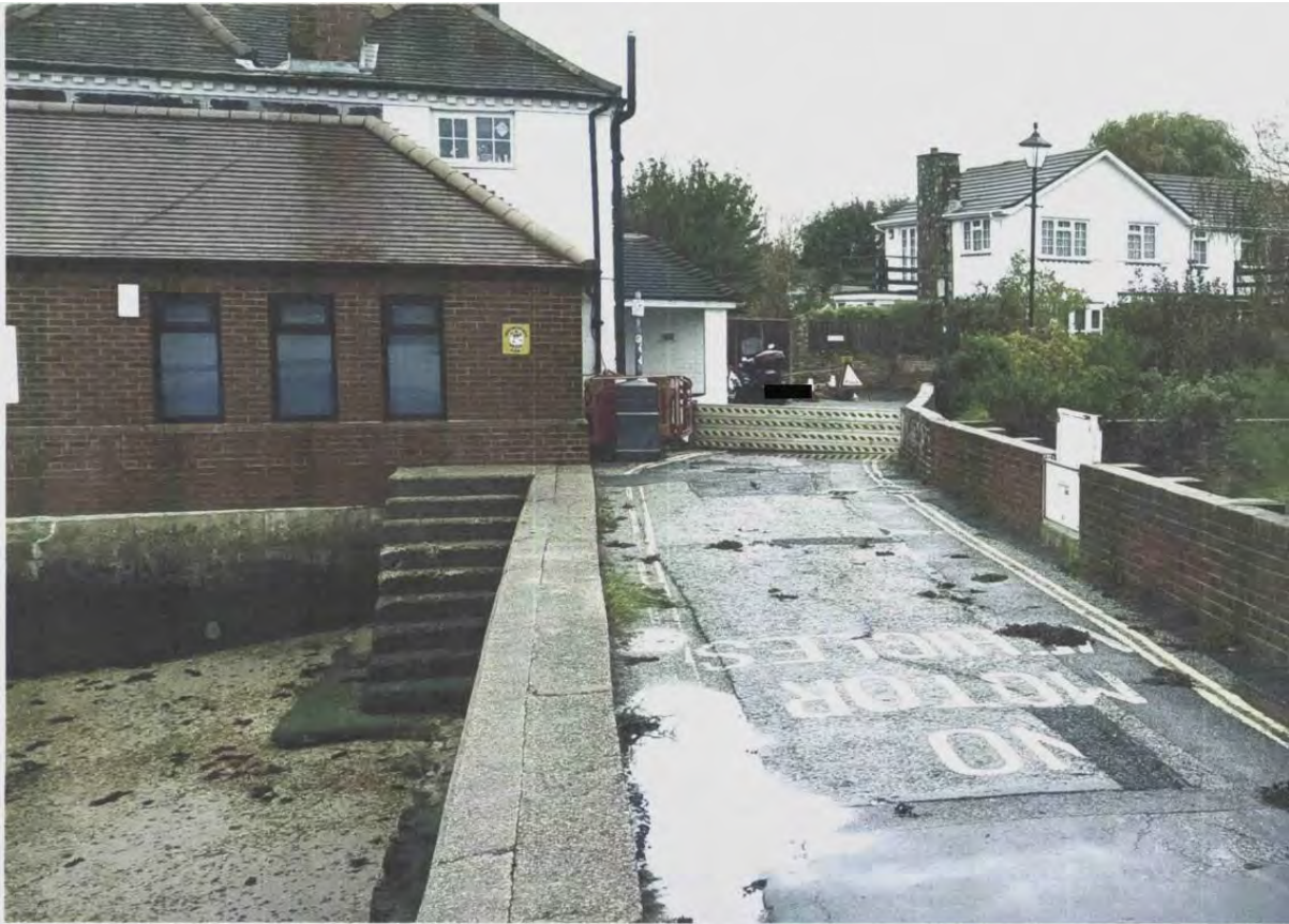
Above: The section of wall (in the foreground) the subject of this application
