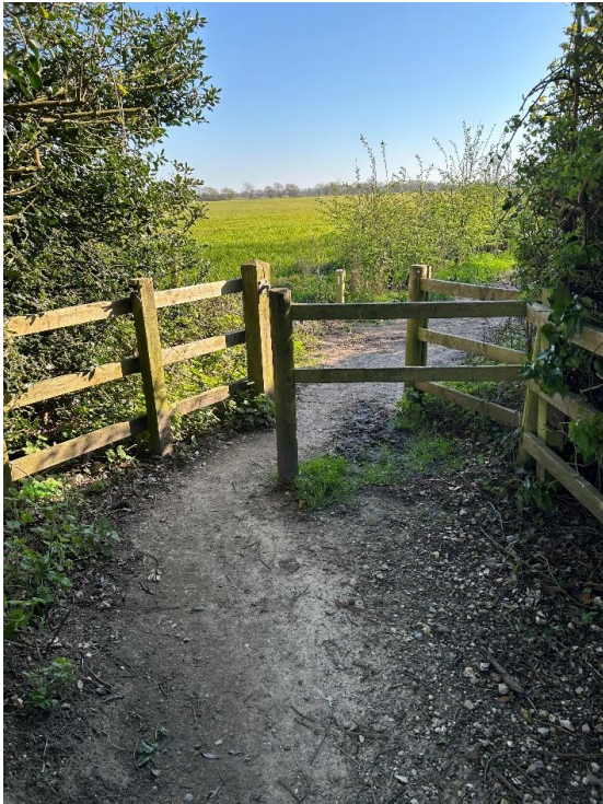
Figure 5. Existing pedestrian gate to be repaired/replaced.
