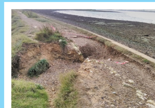
Erosion along a Harbour footpath
