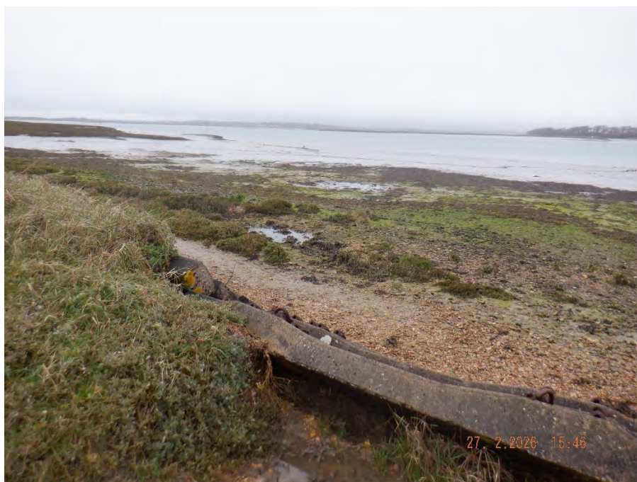
Figure 3.12. Concrete sleepers along the footpath experiencing erosion on the landward side of the sleeper.
