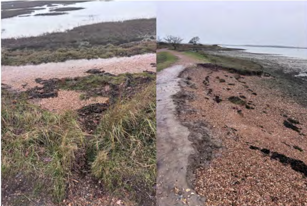
Figure 2.5. Erosion and scour present along the footpath.
